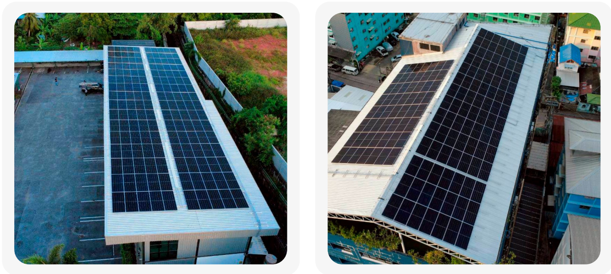
Solar Rooftop at the Headquarters
