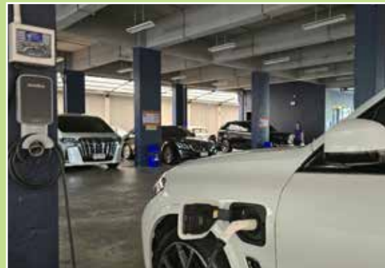
Electric vehicle charging station
